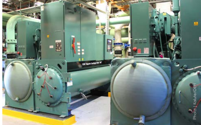
New high efficiency chillers
