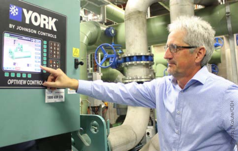
New chiller controls make managing internal climate easy
